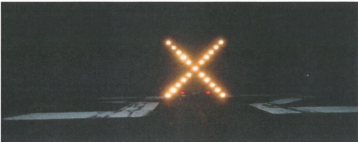
Figure 2-4 Lighted X at Night
