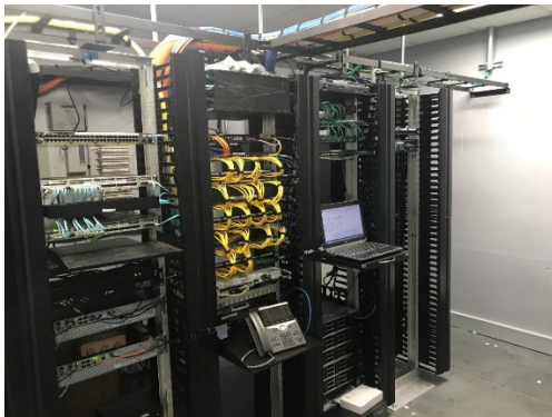
<Photo Example of 4 rack layout>
